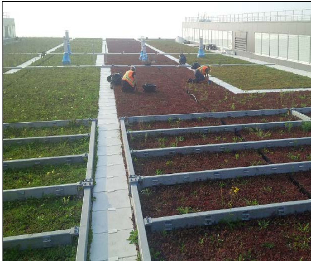
The installation of the Leslie Barns green roof, built to Toronto Green Standards
